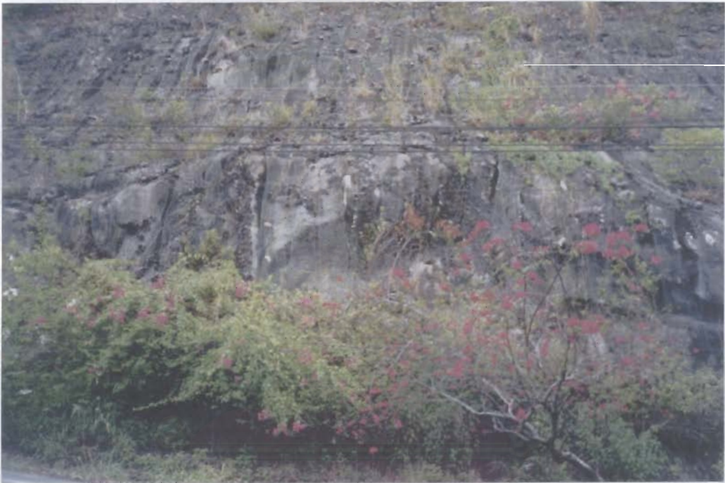
Figure 4.4 Remedy and control the failure along the road between Patong beach-Karon beach, Grid Ref. 232E 640N.
