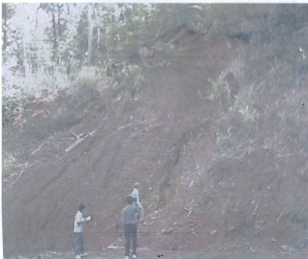
Figure 4.2 Earth slump affected by the highway construction along Highway number 4233 between Kamala beach-Patong beach, Grid Ref. 232E 754N.
