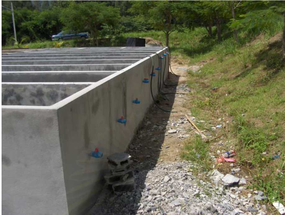
Side View of the FWS Constructed Wetland Outlets
