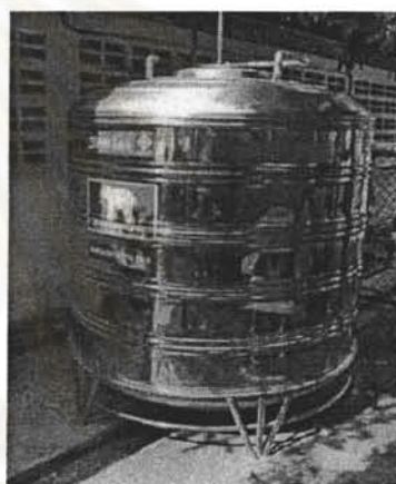
Tank to store filtered drinking water
