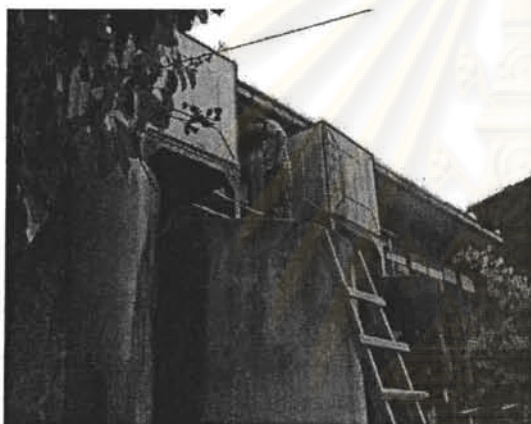
Square-shape tank to store water(underground water)
