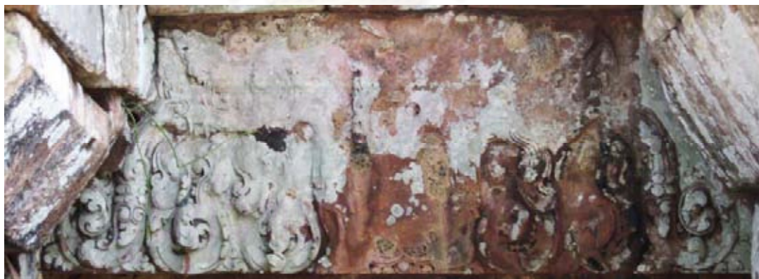
Figure 2- 7: Lintel on the main door (face to the main sanctuary) of the East Gopura. (photo in 2009)
