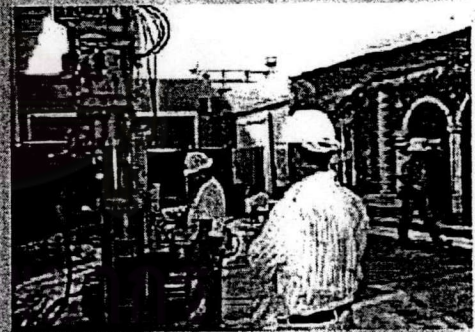
August installing Micropiles at the Clubhouse Restaurant and entrance to the South Coast Plaza in Costa Mesa
