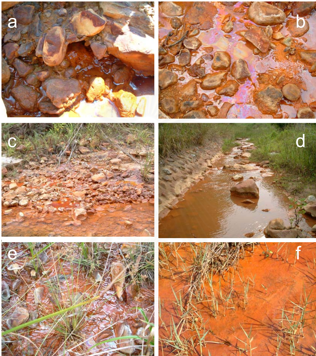
Figure 4.3 Leakage water from the western landfill wall (a). Orange-red leachates from the landfill (pebbles are about 5-15 cm) (b). The leachates flow directly into a natural stream (c). The orange – red leachate downstream (d). Leachate from waste rock built up landfill walls (e). Leachates near landfills and Tum Talu mine at 740754E 691356N (f).
