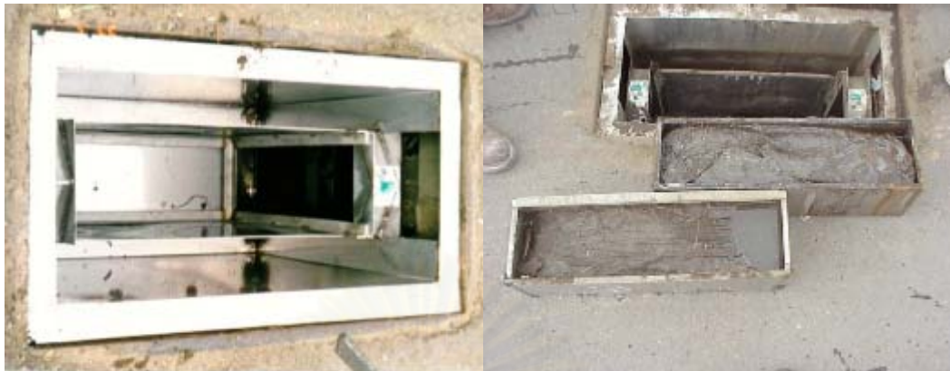
Figure 2.4 AquaShield™ at solid waste transfer station, Knoxville, Tennessee, before and after (Wagner, 1999)
