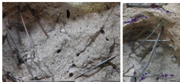
Figure 0-18 COL-B: Hook end embedment in spalled-off concrete
