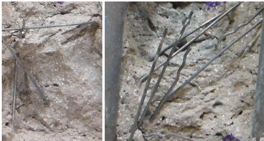
Figure 0-19 COL-D: Hook end embedment in spalled-off concrete
