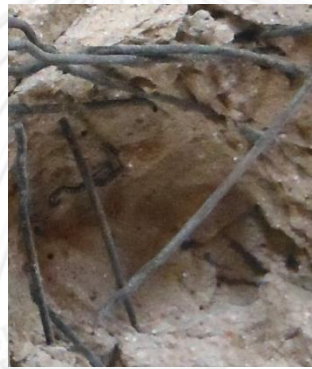
Figure 0-17 COL-C: Hook ends embedment in spalled-off concrete
