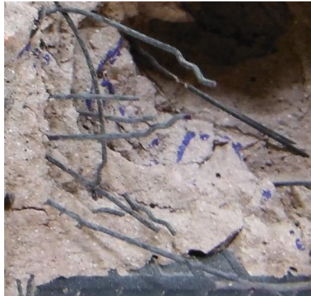
Figure 0-16 COL-C: Cracks running along fiber
