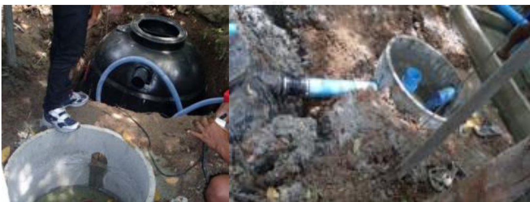
Figure 4-31 Local people are applying a waste grease trap before discharging into main canals (Administration Organization of Bang Nam Pueng sub district, 2011)
