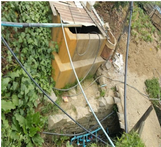
Figure 21 Photo by the Researcher: Water Storage Tank of Private Water vendor and Pipe Allocation by UNICEF in Hakha upland areas
