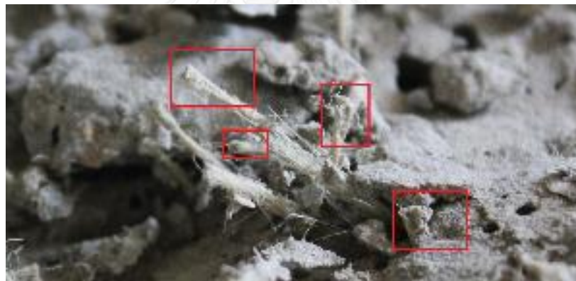
(b) Pull-out failure of 40S specimen
