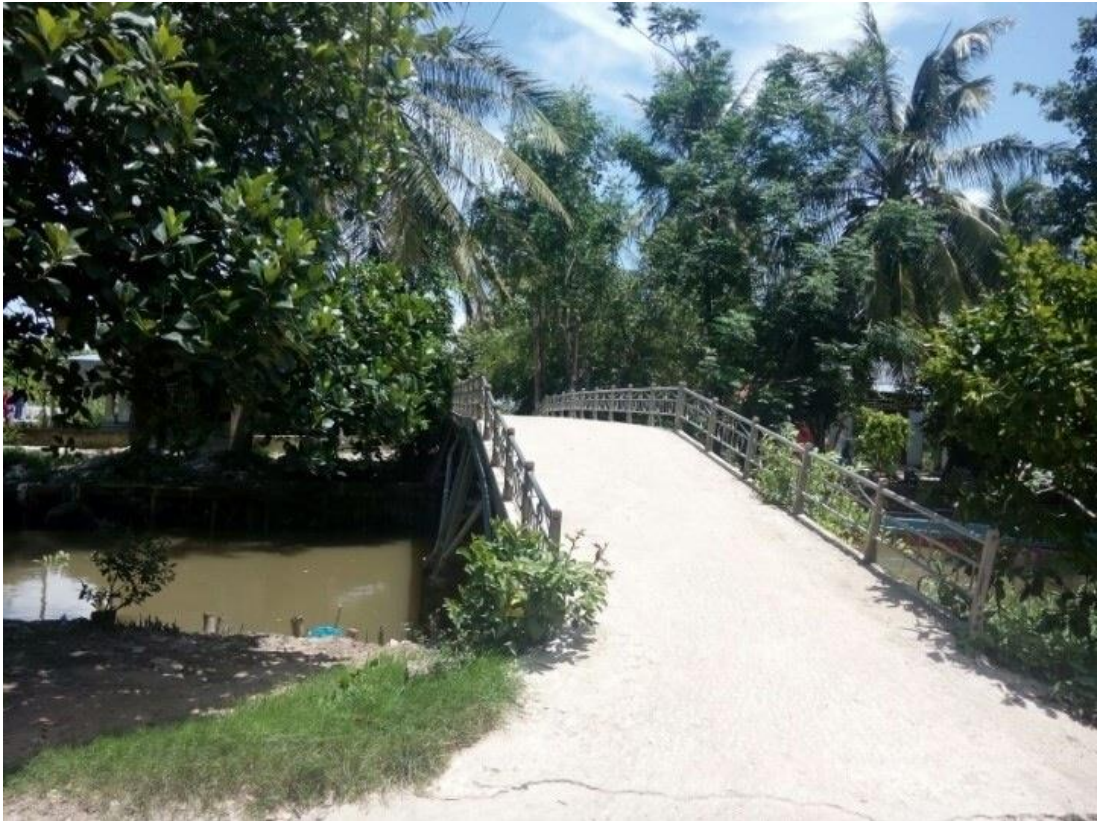
Figure 10: A bridge connecting between Vo Truong Toan and Nguyen Thai Binh Village. The water tanker is not able to cross this bridge to Nguyen Thai Binh Village.
