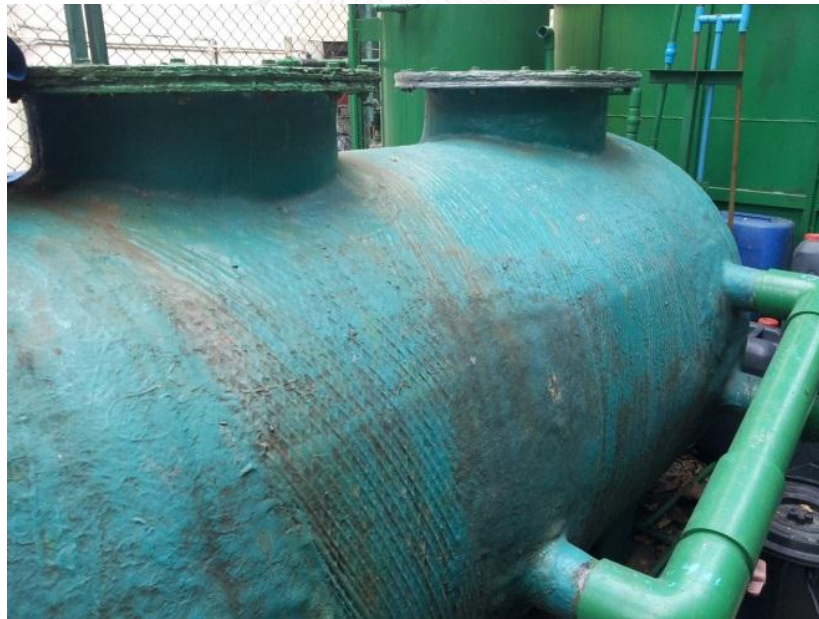
Figure 3.2 Pilot scale single-stage anaerobic digester
