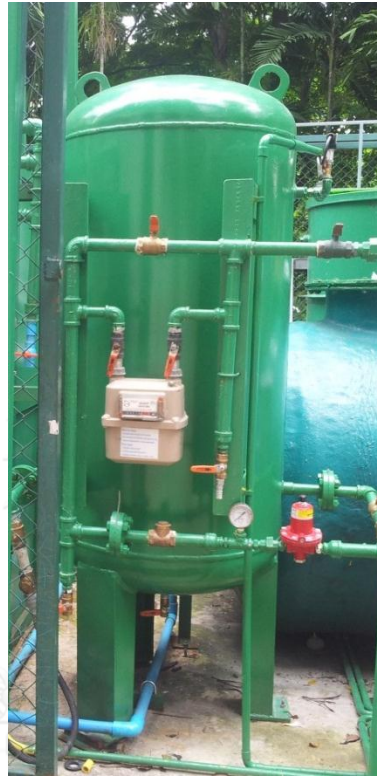
Figure 3.8 Compressed biogas tank
