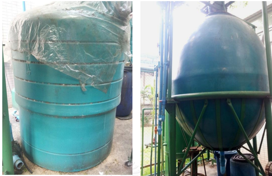
A. Acid reactor
