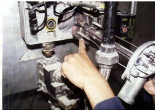
Figure 5.3 The Ignition Electrode of the burner covered with soot
