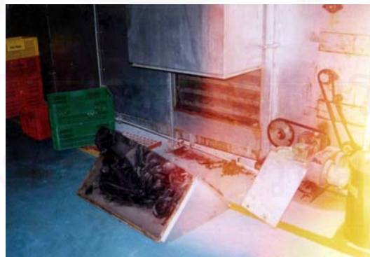
Figure 5.4 The lacking of cleaning of dryer main duct.
