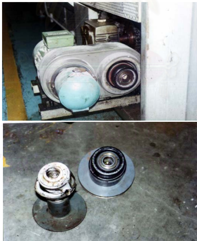
Figure 5.6 The damaged reduce speed control because of lacking of lubrication
