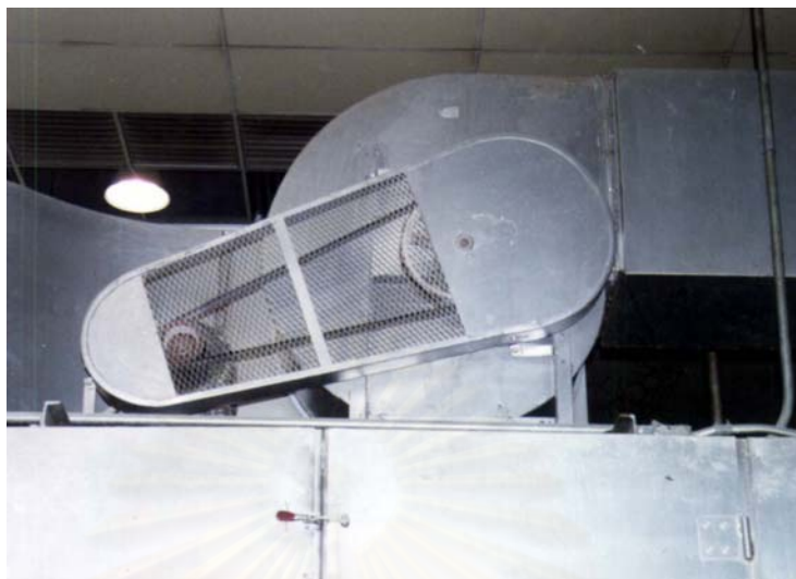
Figure 5.10 The V-Belt of blower that torn
