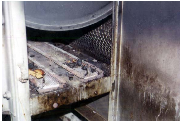
Figure 5.2 The damaged and dirty infrared burners
