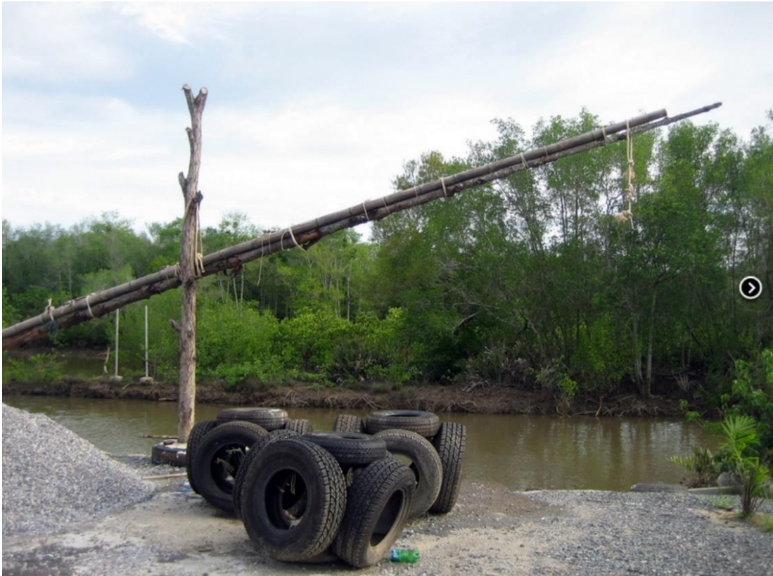
Figure 35. Tire cubes and the crane built with local knowledge Source: website of Ban Pred Nai
