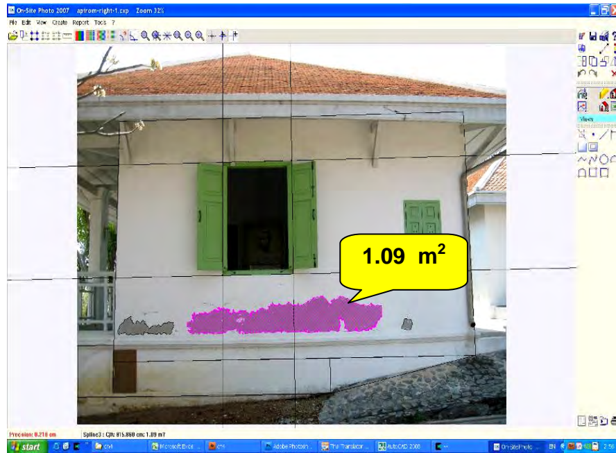
Figure 4.7 The example of damaged area analyzed by image processing
