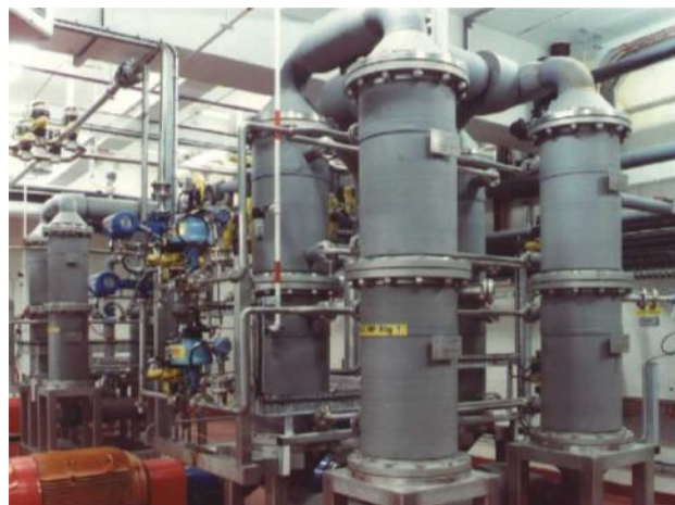
Figure 2.5 Installing the star-shaped microfiltration in GSK plant. [4]
