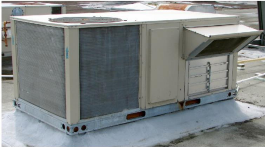
Fig. 45: Self-contained roof-top system [46].
