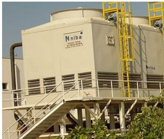
Fig. 31: A Cooling Tower [46].
