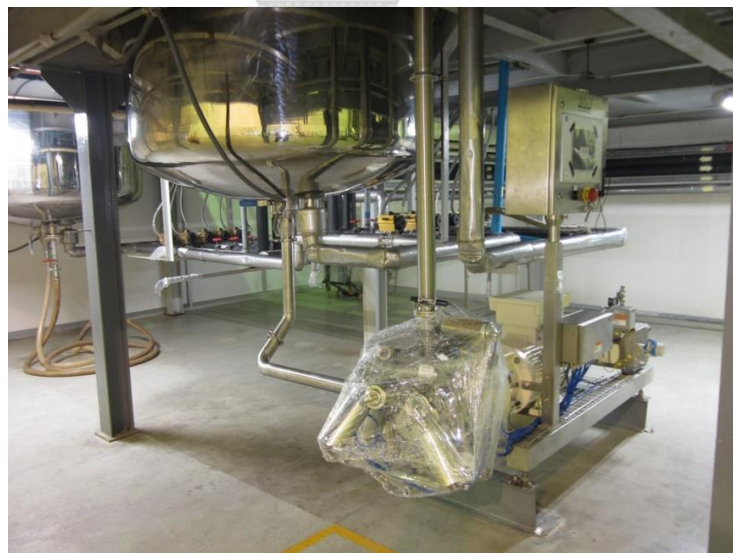
Figure 1-6: Mixing Tank for 2,000 L
