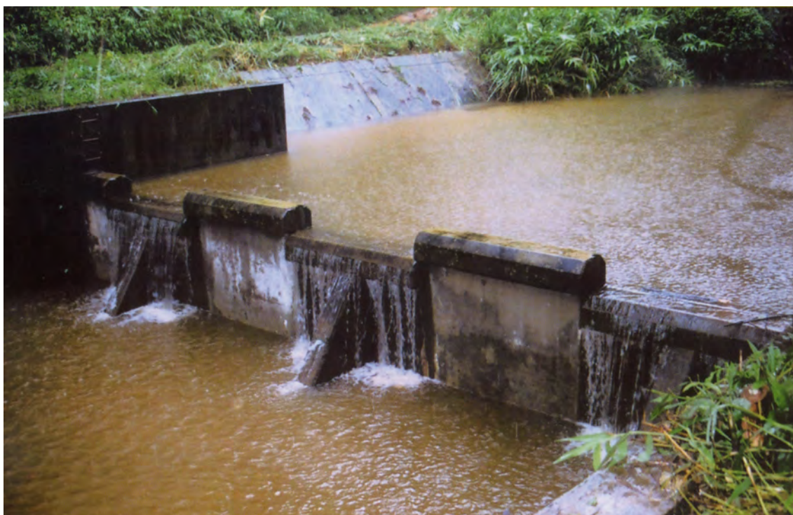
Dam in Nong Hoi village, Mae Rim district, Chiang Mai, constructed following the ideas of King Rama IX
