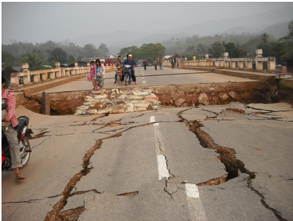
Figure 1.3. The photo shows the damage established by The M_w -6.8 Tarlay earthquake on March 24 th , 2011, in Myanmar. ( https://upload.wikimedia.org )
