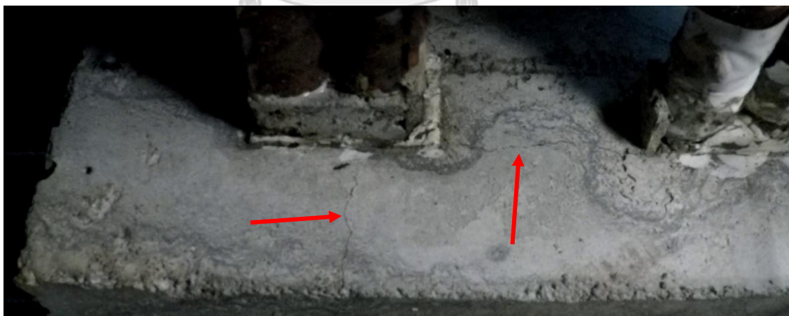
Bottom splitting cracks and between lapped bars (L28C2SC)
