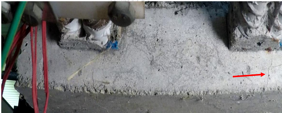
Bottom crack first (L28C1SC)
