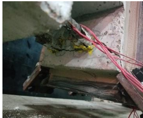
(b) Splitting cracks restrained (Type-III)
