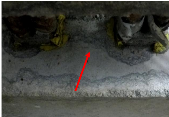
(1) Splitting between lapped bars
