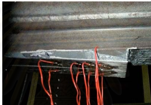
Figure 7.1 Premature separation of bonded CFRP plates from the steel beam
