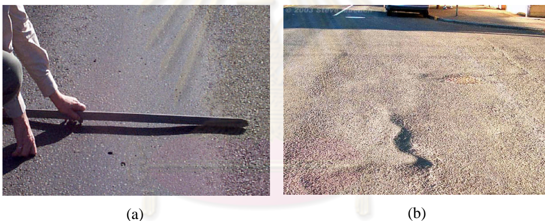
Figure 2.2 (a) Distress of rutting (b) Distress of shoving
