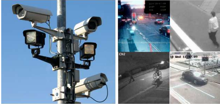
Figure 5.1: Fixed CCTV camera above junction road.
