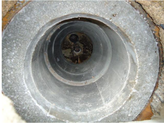
Figure A.5: The new casting cement inside the kiln with low-cement castable type: D59A
