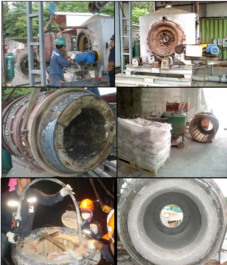
Figure A.9: The reparation of the pilot-scale rotary cement kiln for casting new cement inside the kiln with low-cement castable type: D59A
