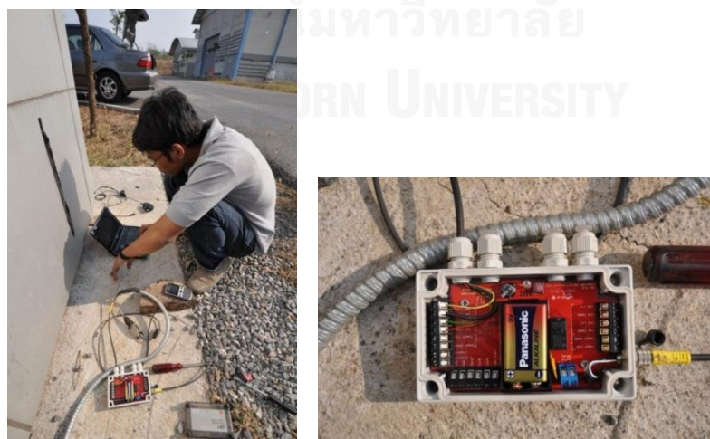
Figure 3.25 Equipment Control and Maintenance
