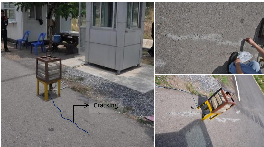
Figure 4.19 Occurrence of Cracking in Site 1 & Reparation Using Asphalt Binder
