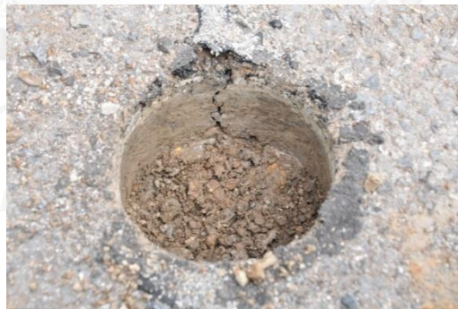
Figure 4.20 Cracking on Observation Point of Site 1
