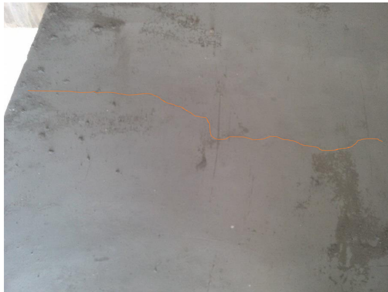
Figure 4.17 Cracks in wall resulting from lack of skilled labors
