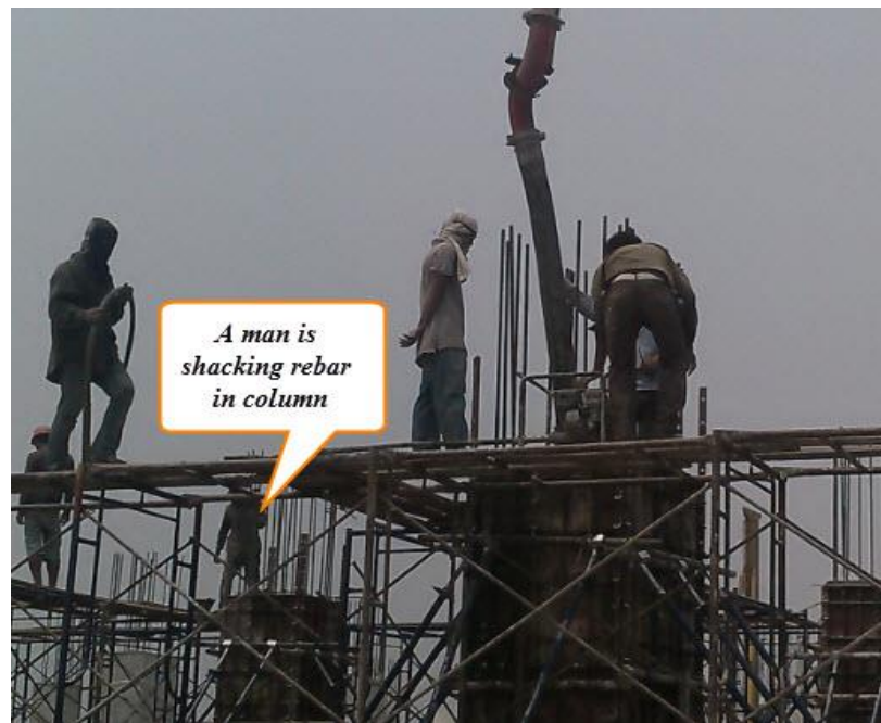
Figure 4.13 A wrong technique of column concrete pouring
