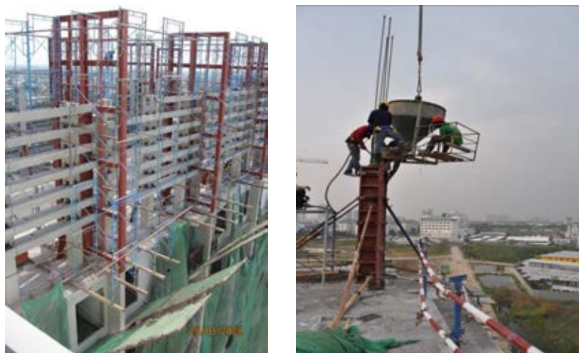
Figure 4.3 Existing falling object hazards from sample project number 1 and project number 3
