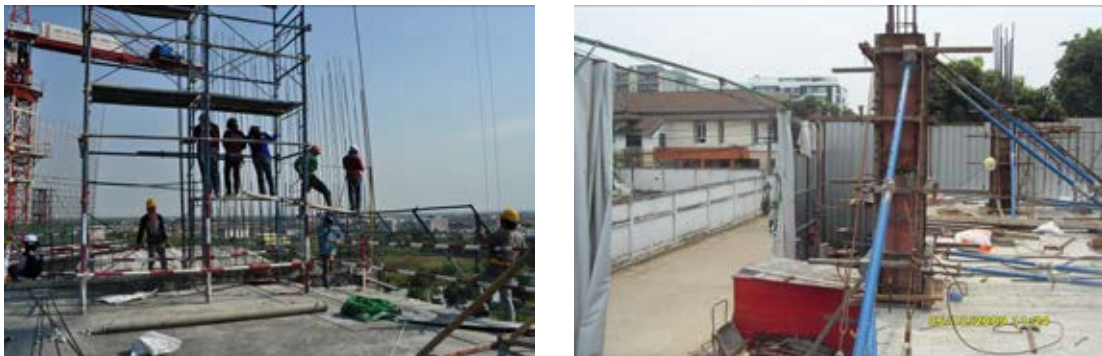
Figure 4.12 Unsafe work areas
