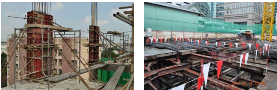
Figure 4.2 Existing fall hazards from sample project number 4 and project number 5
