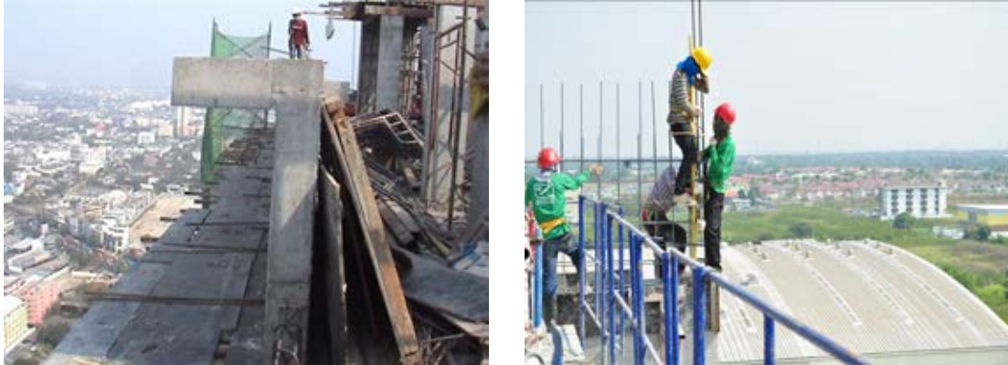
Figure 4.1 Existing fall hazards from sample project number 2 and project number 3
