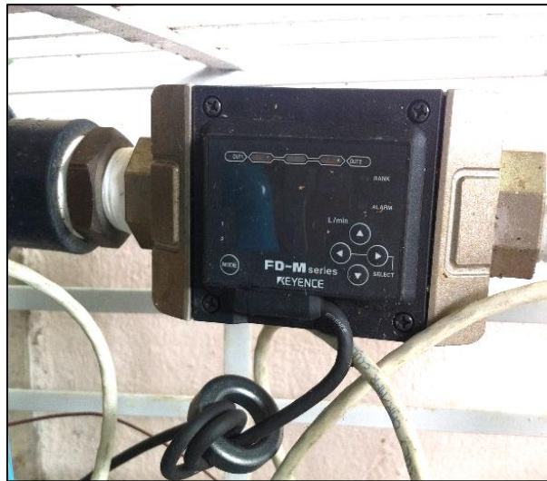
Figure 2.8 Flow meter for flow rate.
