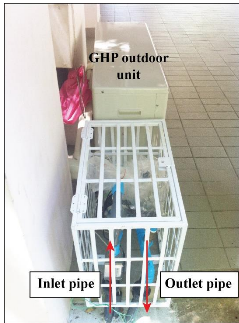
Figure 2.21 Connecting HDPE pipe from well nos. 1&2 to GHP outdoor unit.
