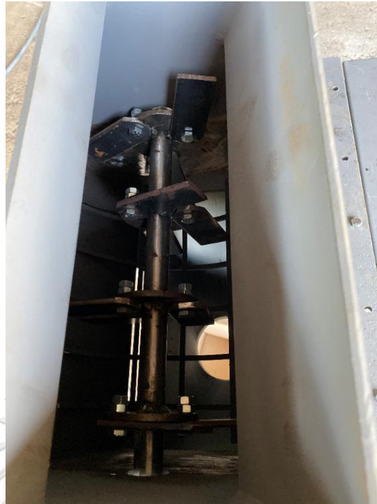
Figure 45: Top view of hopper
