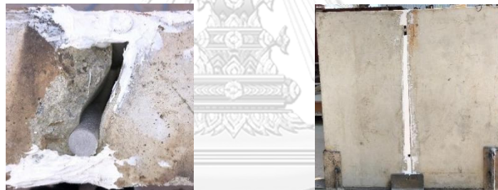
Figure 39 The top view image (left) and front view image (right) of a scarfs drains joint.
