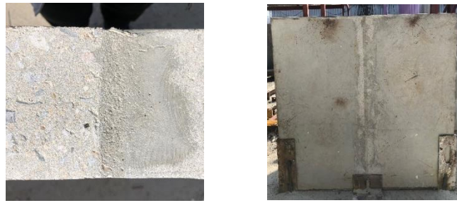
Figure 38 The top view image (left) and front view image (right) of a one-stage joint.
