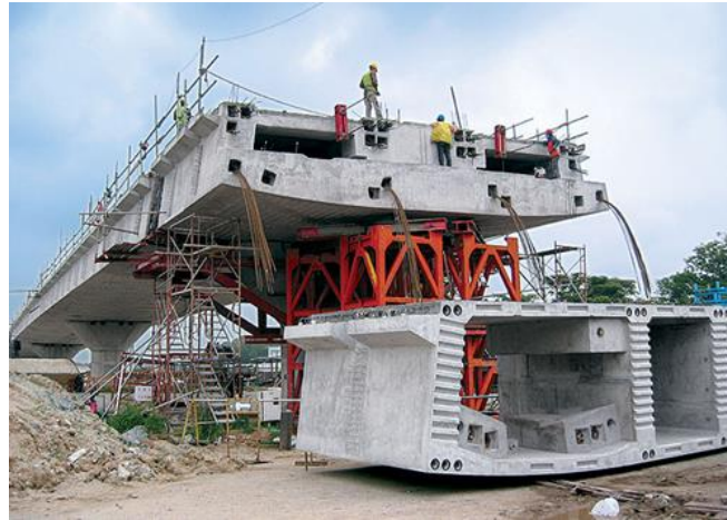
Figure 2-1 Construction of concrete segmental bridge fabrication from Airport Road to Tampines Avenue 10, Singapore
