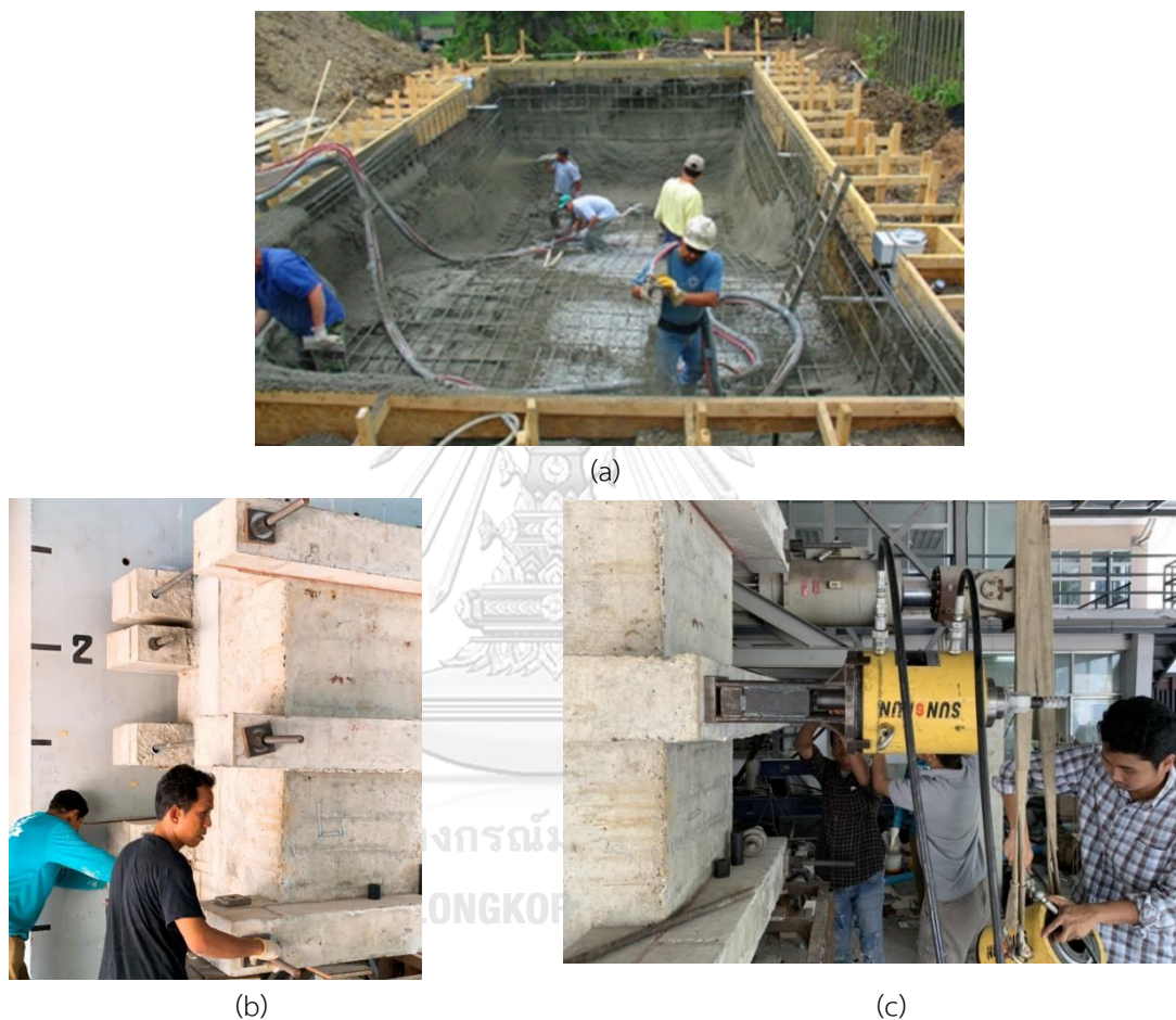
Figure 5-9 Comparison of swimming pool working process between traditional system and our precast system; (a) working process of traditional construction system; (b) and (c) working process of our precast construction system
