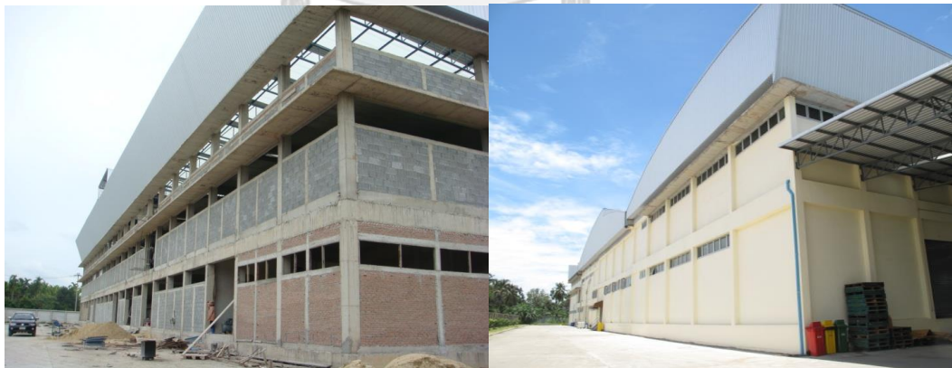
Figure 5-1 Our previous construction work on a 16000-sq.m. food plant at Bhuddamonton sai 7
