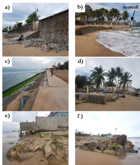
Fig. 8. a) Seawall at Had Pran Khiri (Z3), b) Shoreline erosion in Z3, c) Seawall along with Laem Ket (Z4), and d)-f) Property damages between transect 134 – 140 (Z4).
