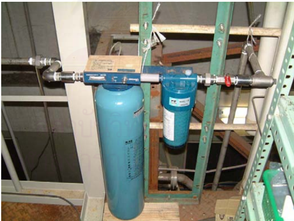
Fig.4.10 Make-up water pipe
