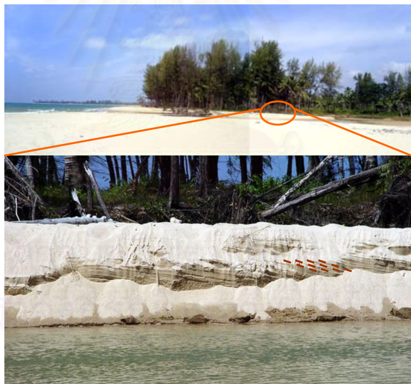
Figure 4.63 Photograph showing new backshore sediment indicate inclination of layer in landward direction (looking north) deposited where eroded channel back occurred.
