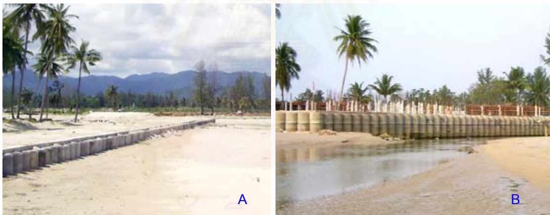
Figure 4.45 Photographs showing new sea wall was constructed parallel to the shoreline (A) and sea wall along the tidal channel (B).
