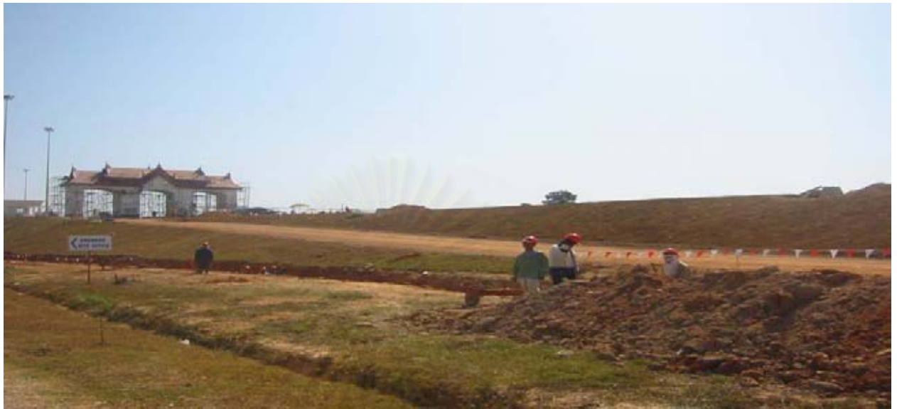
Figure 6: Route 9 road Savannakhet - Construction of the boarder administration area that will process vehicles that have entered Lao via the newly constructed Second Mekong Friendship Bridge.
