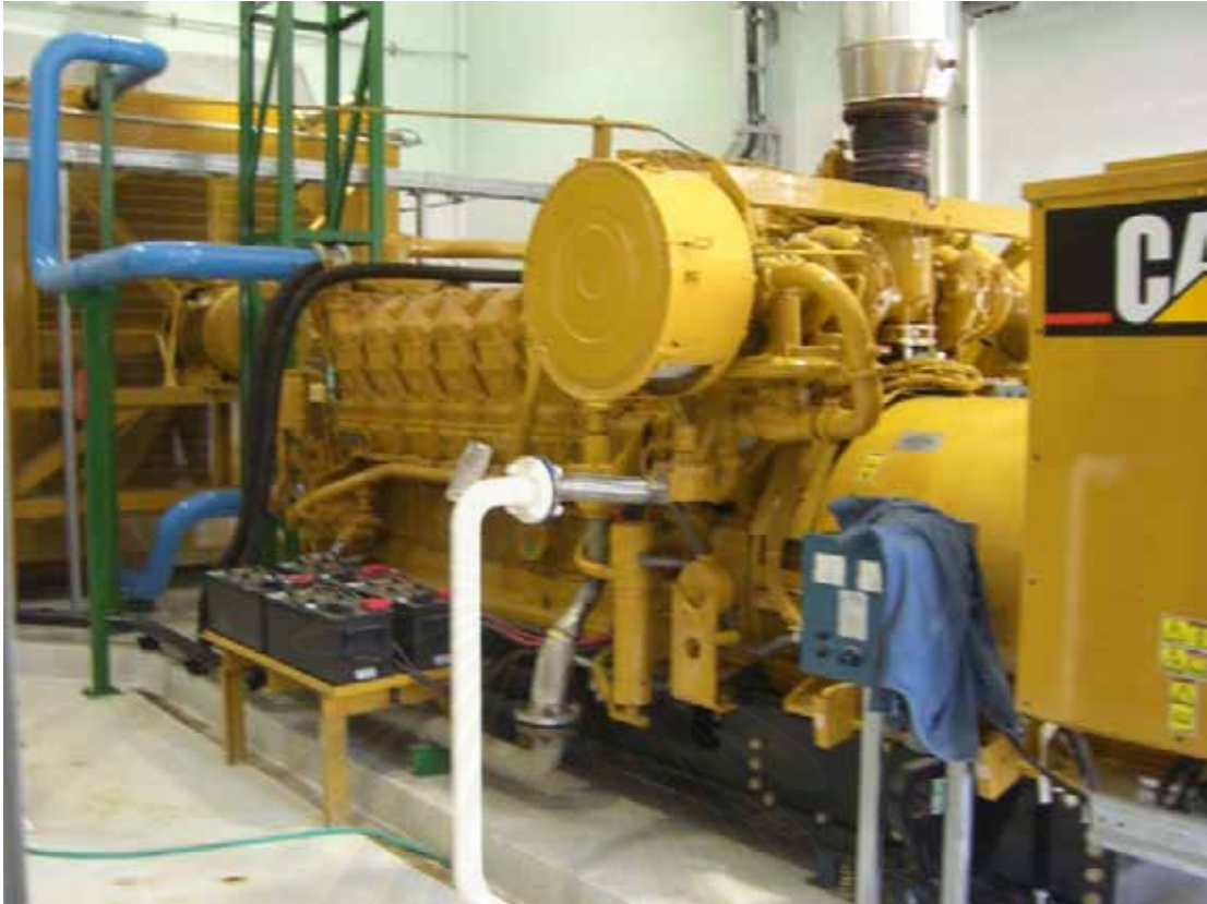
Figure 4-2 Gas power generator
