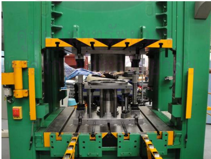
Figure 7.12 Die installed in press machine
