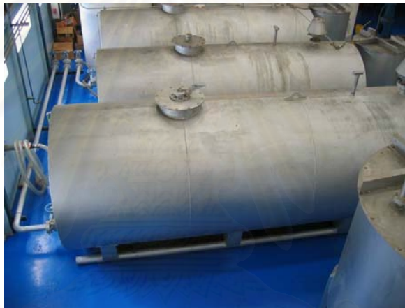
Figure 3.10 Base oil tanks
