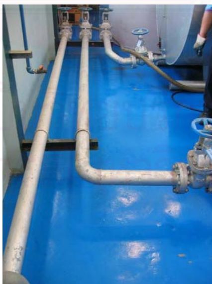
Figure 3.14 Valves and pipes of base oil tank
