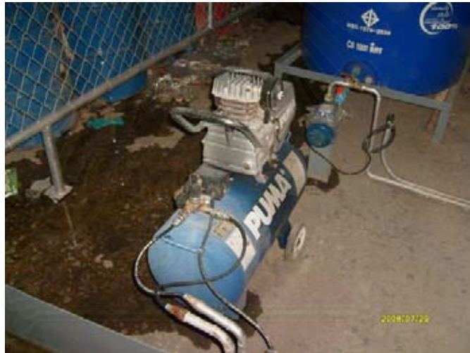
Figure A-7 Air pump for control spray of the water in cooling tower
