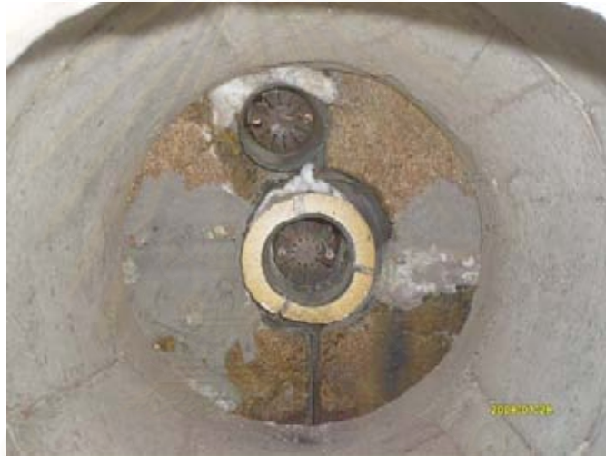
Figure A-4 New casting protected heat cement inside the kiln and two burners
