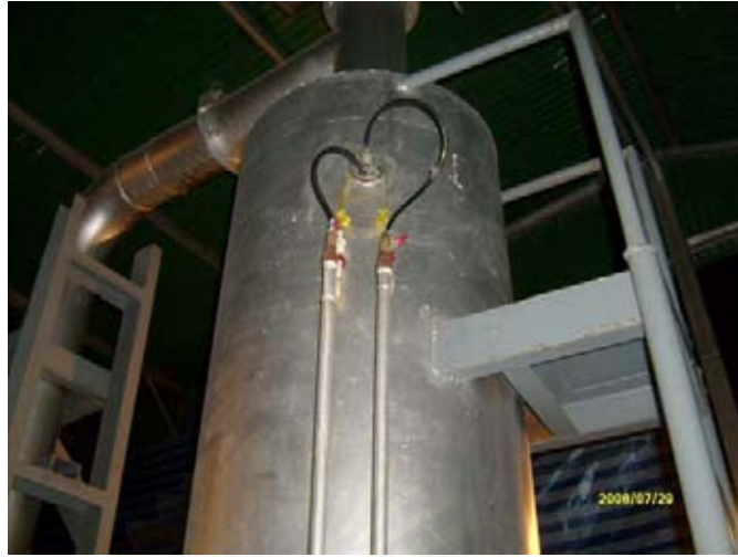
Figure A-6 Cooling tower
