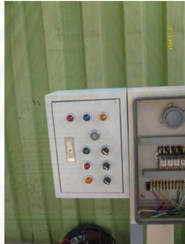
Figure A-10 Control boxes
