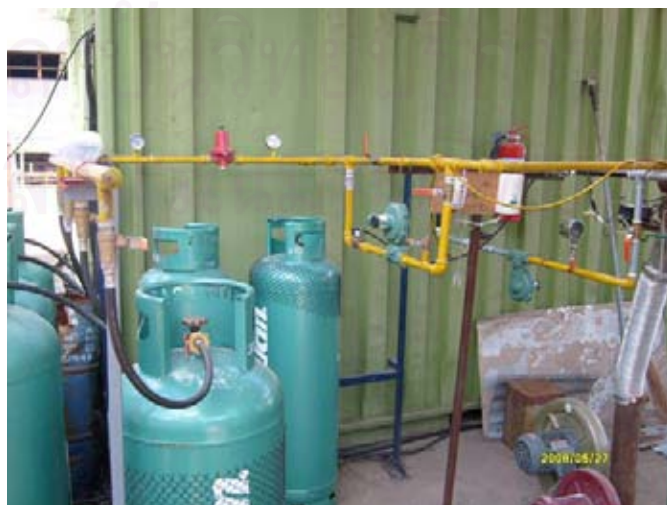
Figure A-8 Gas station and pressure control
