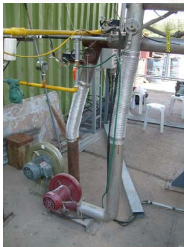
Figure A-5 Two blowers
