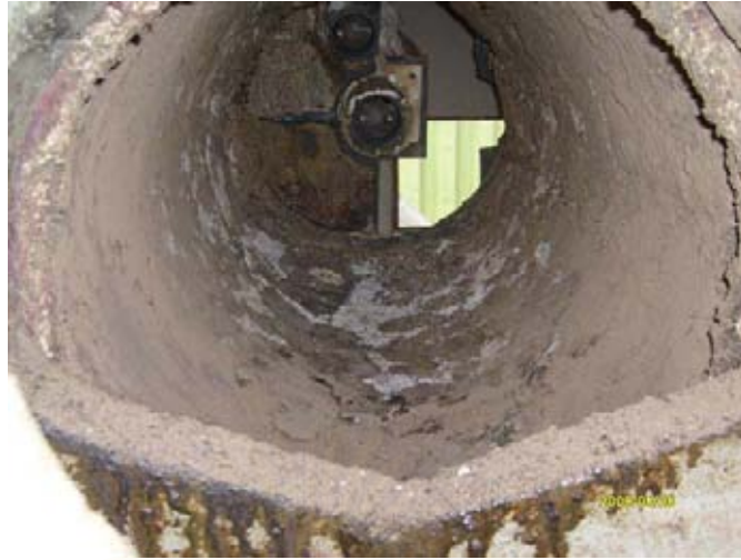
Figure A-3 Damage inside the pilot scale rotary cement kiln
