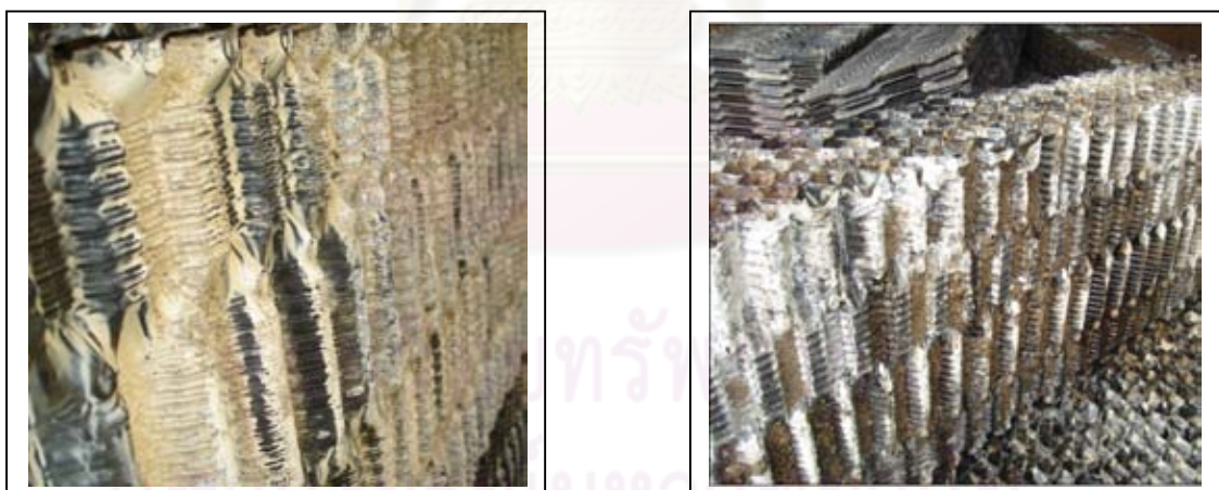
Figure 2.5.1 (a) and (b) show the fouling problem (90-95%) in fill pack CW#1 and CW#2
