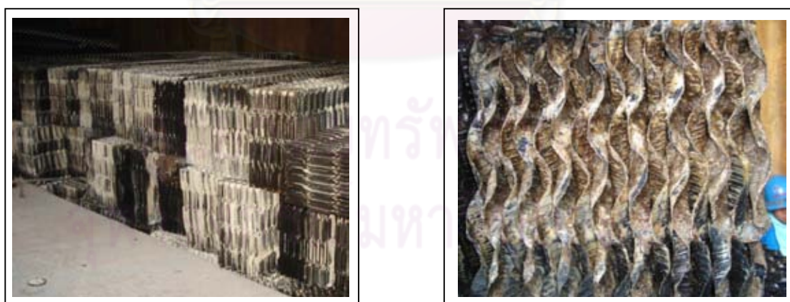
Figure 2.5.4(a) and (b) shown the fouling problem (90-95%) in fill pack CW#7 and CW#8
