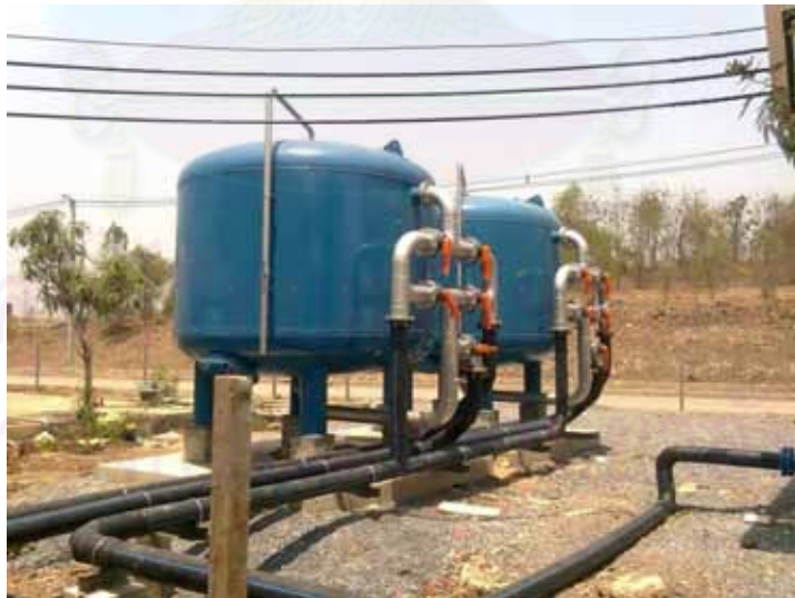
Figure A-4 Sand Filtration Unit
