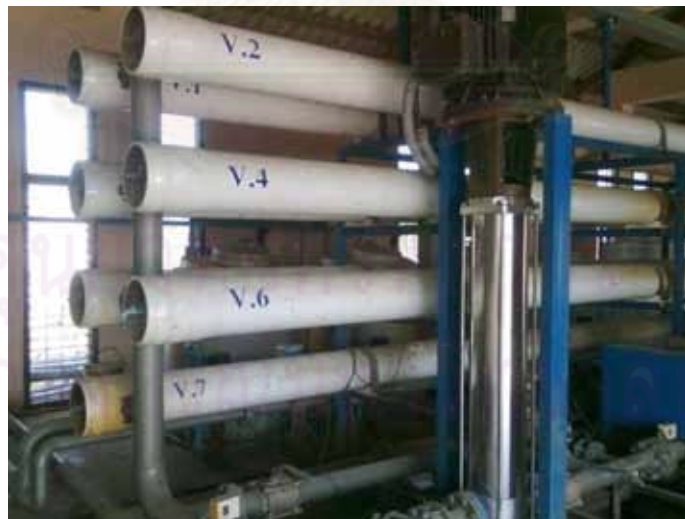
Figure A-6 Reverse Osmosis (RO) unit
