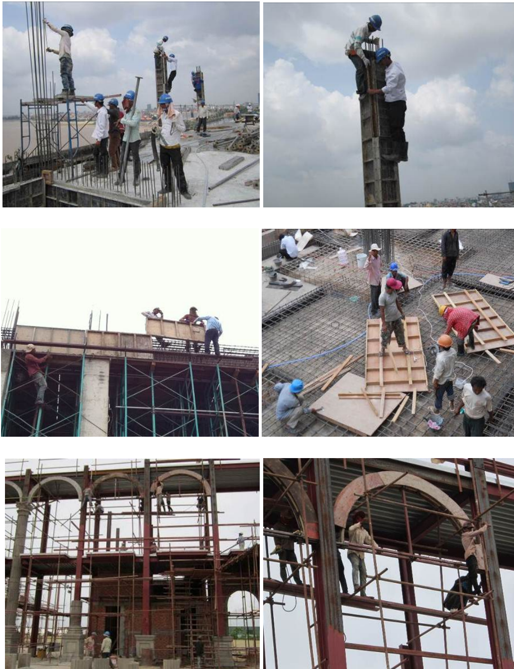
Figure 4.12 Site observation shows improper use PPE by workers (local contractors)
