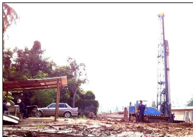
Position of foreman, labourer and machine operator in drop hammer piling operation
