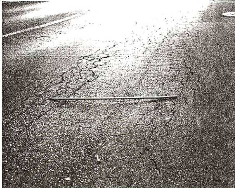
Figure 2.3 Rutting along the wheel path in HMA pavement.[6]
