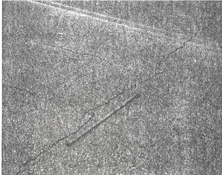
Figure 2.5 Transverse cracking due to temperature change.[6]
