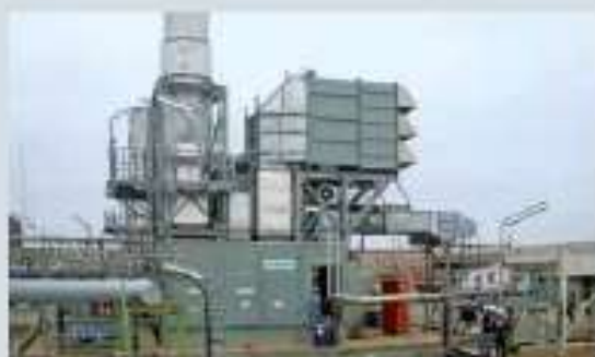
Sasol Technology (Pty) Ltd, South Africa: The 13.4MW SGT-400 gas turbine is the key component to the two pipeline compressor sets installed at the Komatipoort compressor station.
