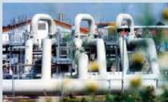
Wingas compressor station, Eilschieben, Germany: Two Siemens compressor trains, each powered by a 30MW SGT-700 gas turbine, boosting the pipeline pressure for Natural gas* transport.
