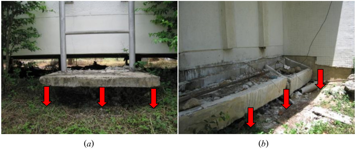
Figure 3.4 (a) shows the side step of the building separated from the ground. (b) shows cracks on the sidewall of the same building.
