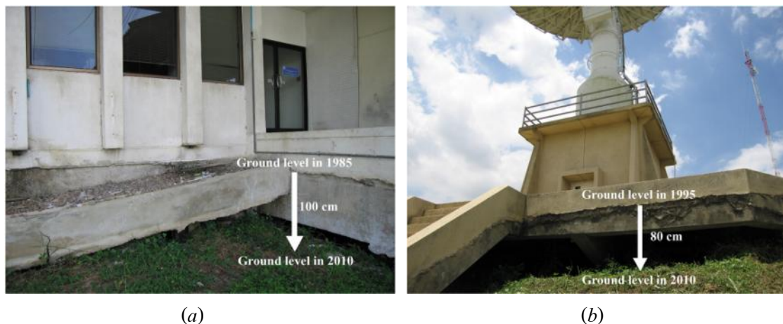
Figure 1.2 Gaps opened due to differences between subsidence of the ground surface and buildings whose foundations rest on the sand layer found at earth observation center located near Ladkrabang district, Eastern Bangkok.
