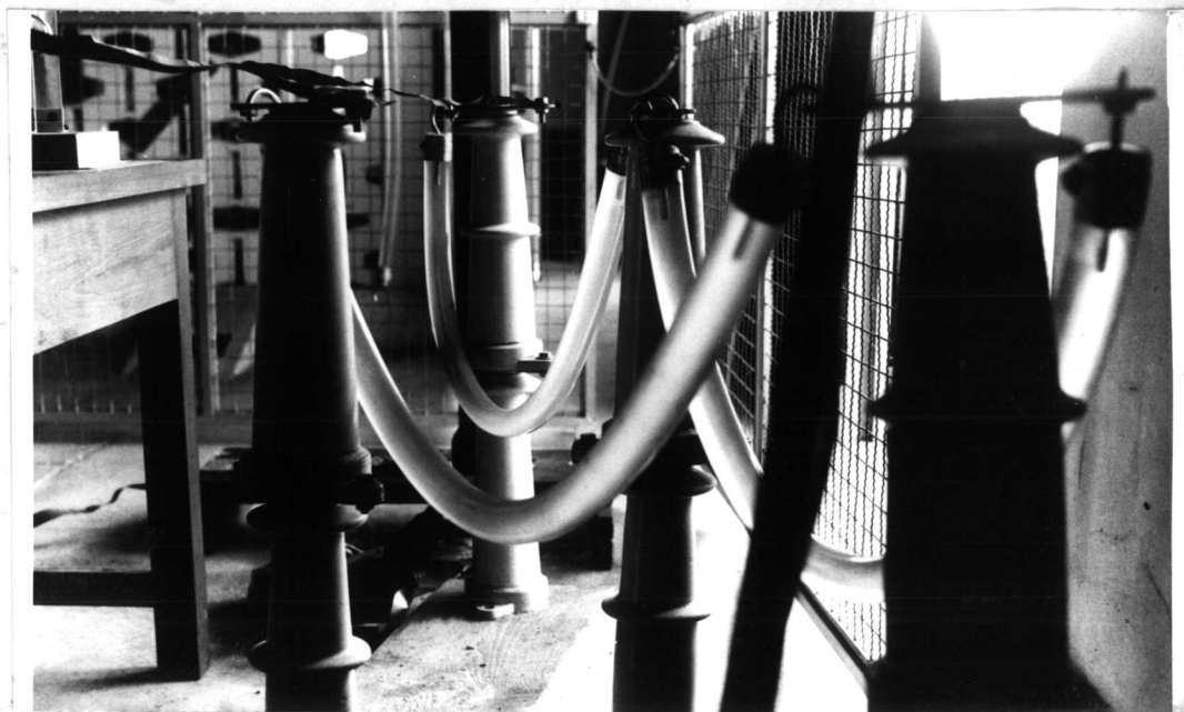
Fig. 3-12 Liquid Resistors used as the limiting resistances of the voltage doubler circuit
