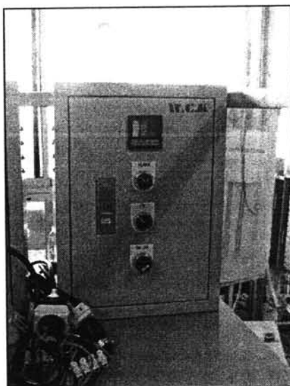
Figure 3.7 The temperature control box.
